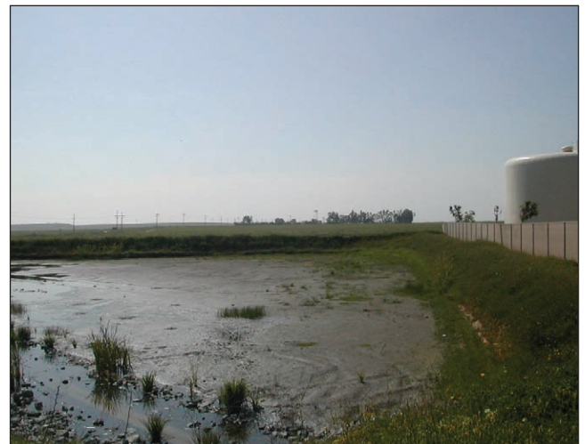
Stormwater drainage facilities on the project site include an approximately 3.9-acre rectangular detention basin, located between the fire station and wastewater treatment plant.
